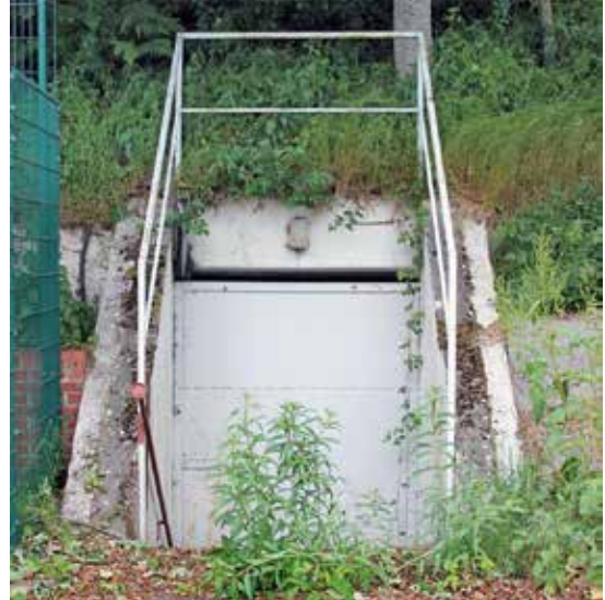
External view of emergency exit from car park level. Door was part of the original WWII SOC bunker
